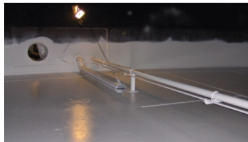
Interior crude oil storage tank
